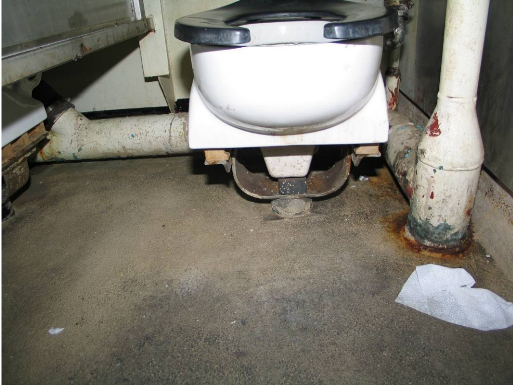
The deck coating and the coving surface are 100% intact and the rust observed on the Durabak is stain only. The uneven texture of this application is apparent in this photo
