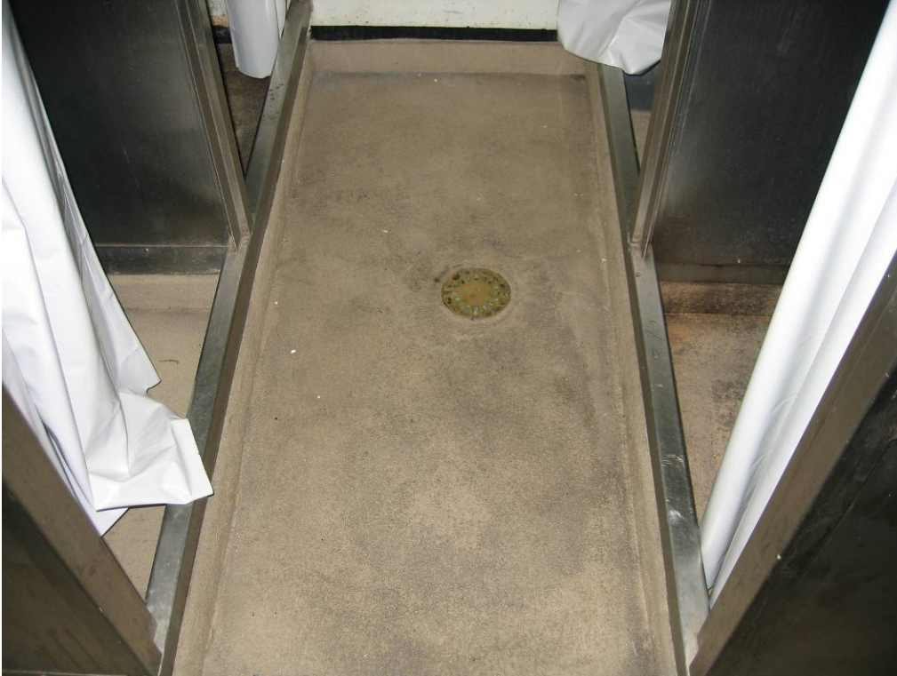
The perimeter around all deck drains throughout the washroom is in excellent condition
