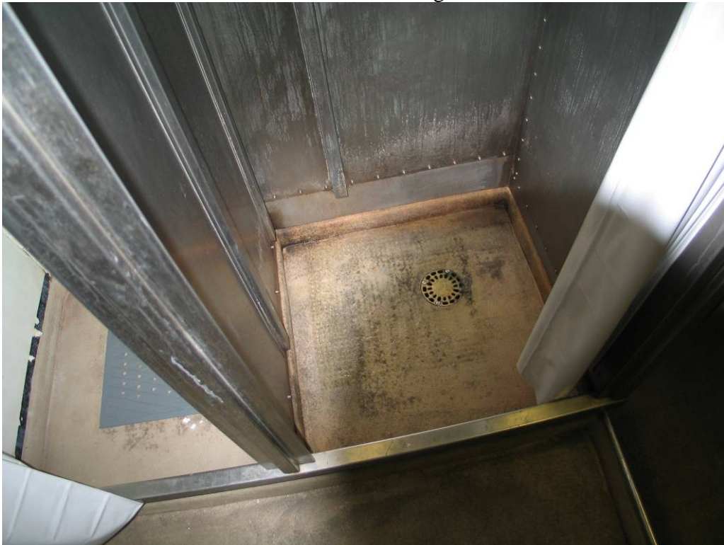
Shower stall mold and mildew. The deck coating and coving are in excellent condition. The perforated bath mat was lifted out of the way for the photo. The mat had a heavy slime on the underside.
