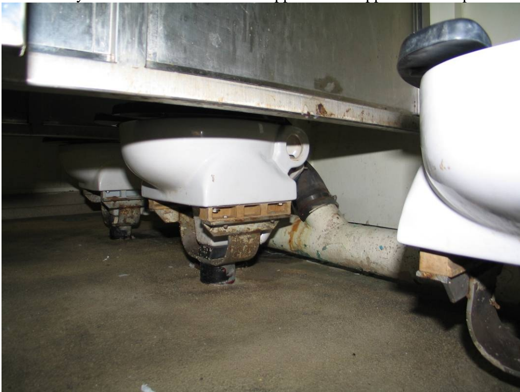
This configuration makes proper cleaning problematic.
