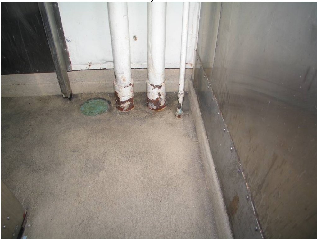
The somewhat uneven texture of this application is not unacceptable but proper application technique with this material is possible and results in a more even texture.
